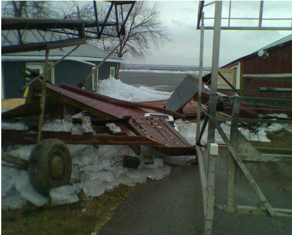
Rising water levels combined with wind drives ice into south side cabins on Lake Poinsett
