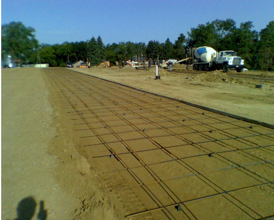
Beginning to pour concrete floor of 600 head monoslope feeding facility with manure storage containment
